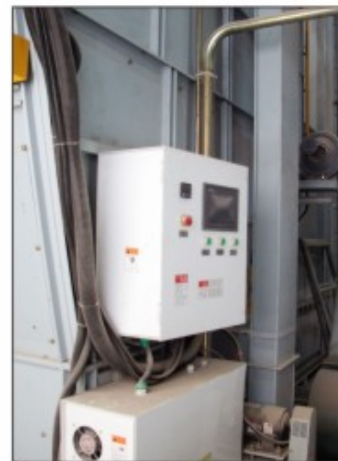
稻壳炉控制系统 STOVE ELECTRICITY CONTROL SYSTEM
